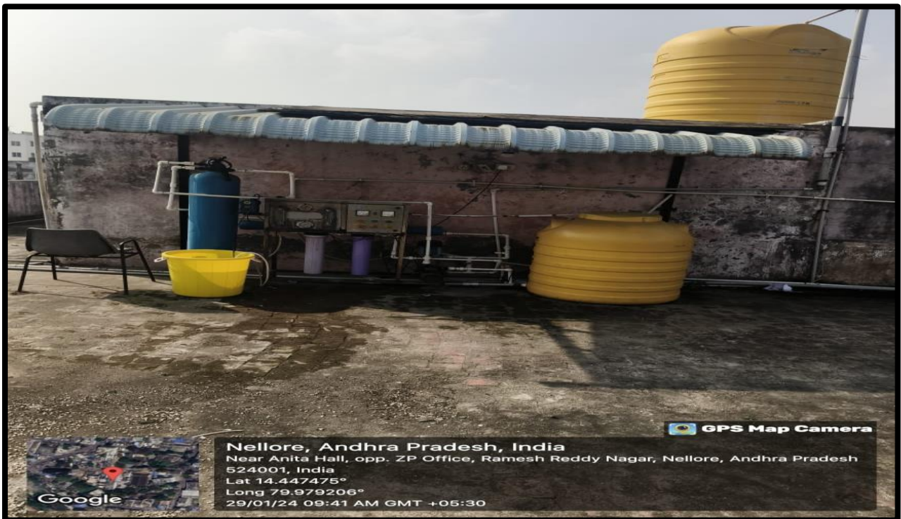
Figure: 2: RO System Control Panel with Storage Tanks at KCDC Campus
