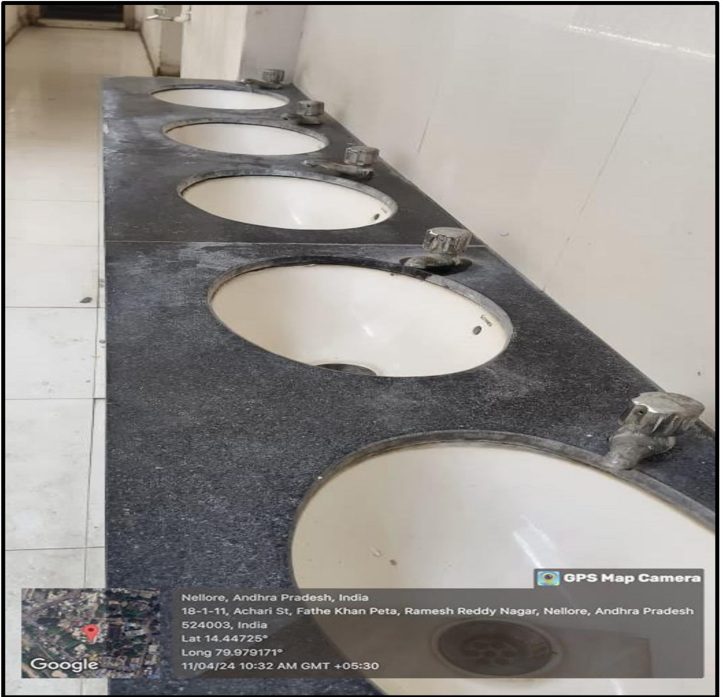
Figure 2: Usage of Waste water for hand wash
