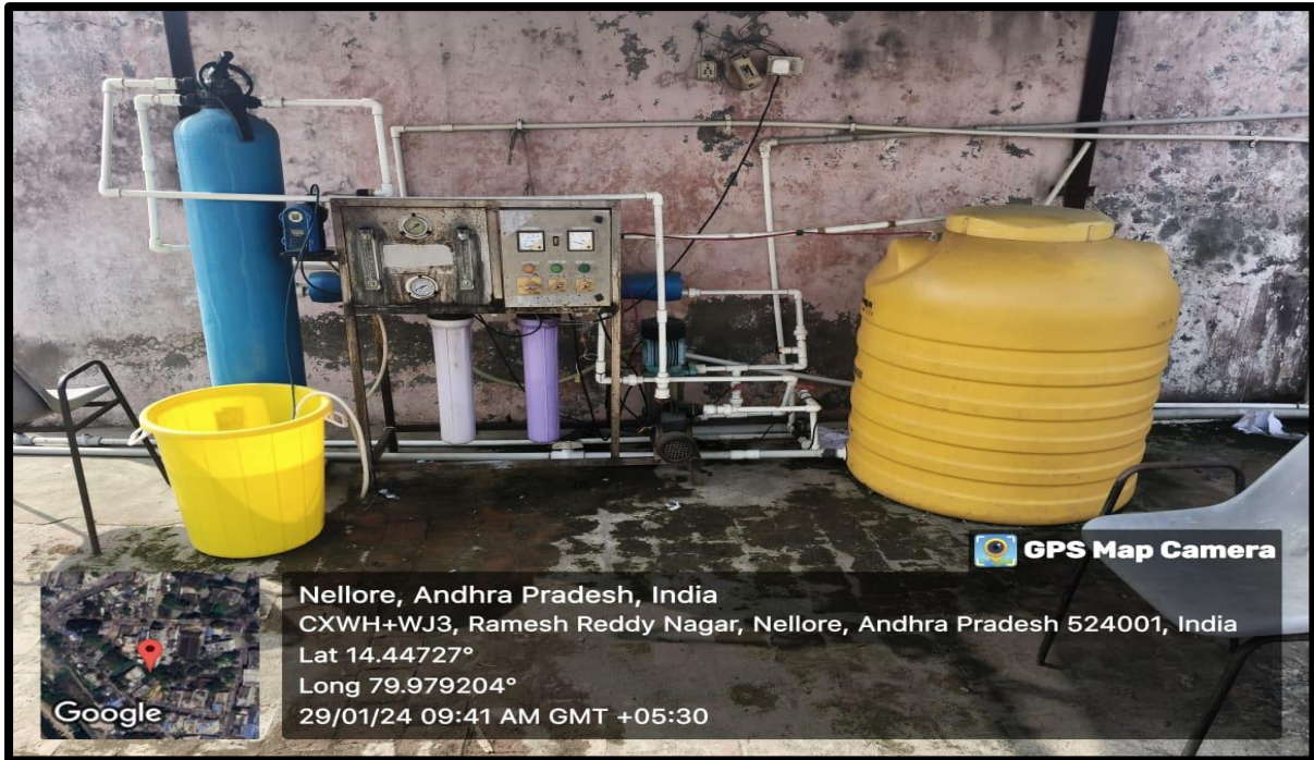
Figure: 1 RO System Control Panel with Storage Tanks at KCDC Campus
