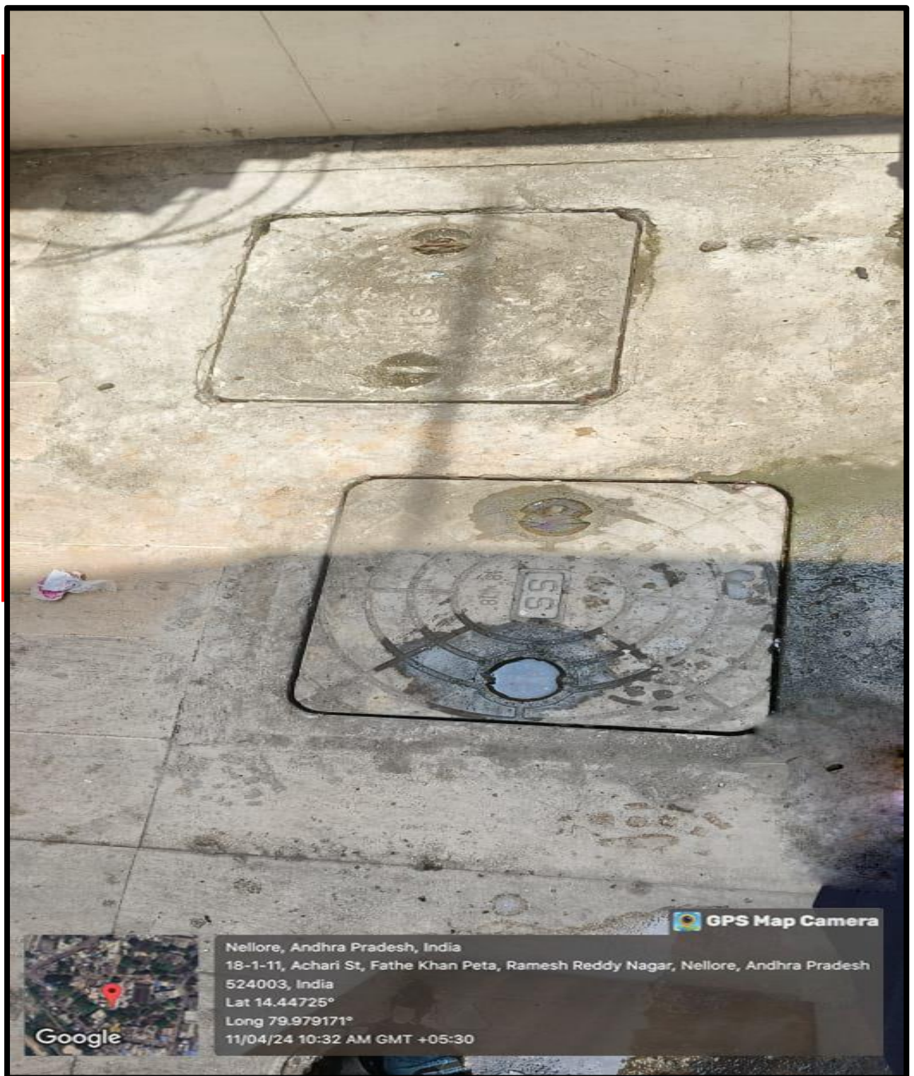
Figure: Water storage sump/Tank front part
