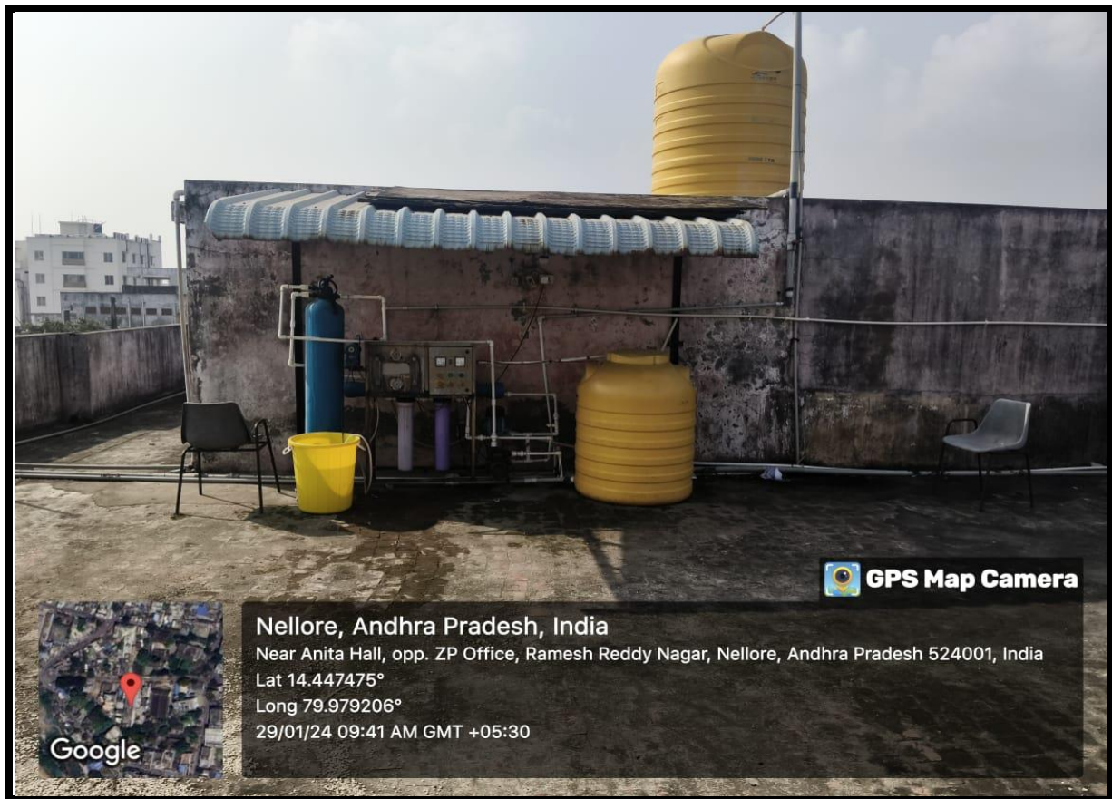
Figure-1 Water Tanks
