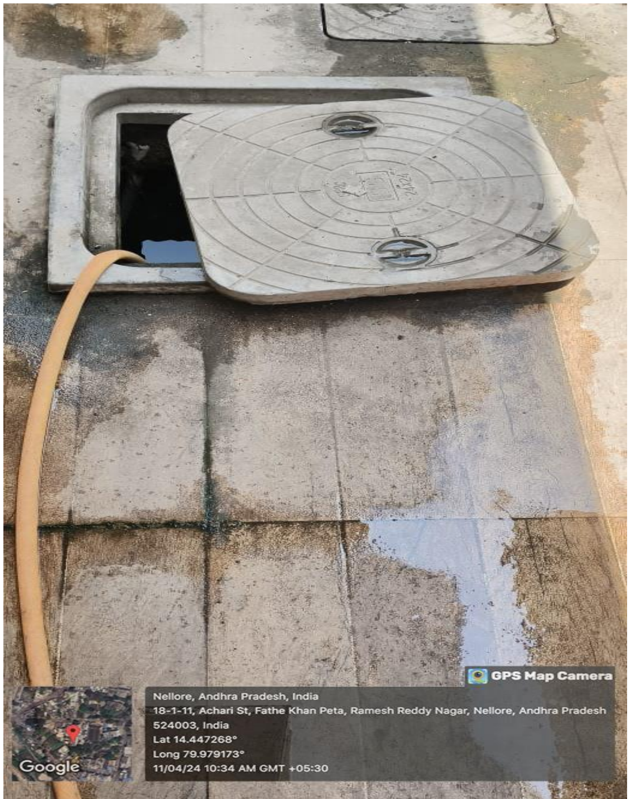
Figure: water Storage Sump/Tank Outer Portion
