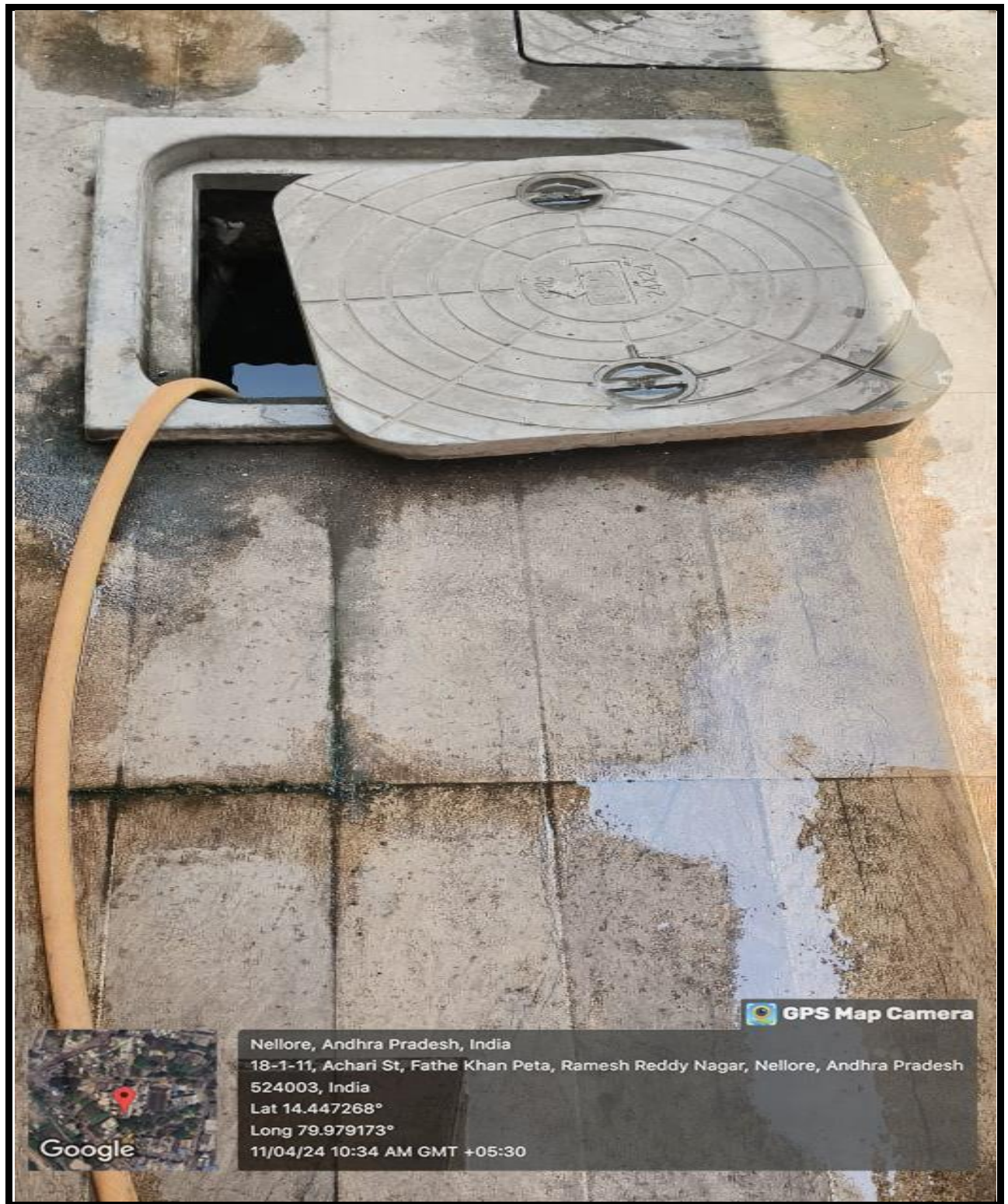
Figure: Water Storage Sump/Tank Inner Portion
